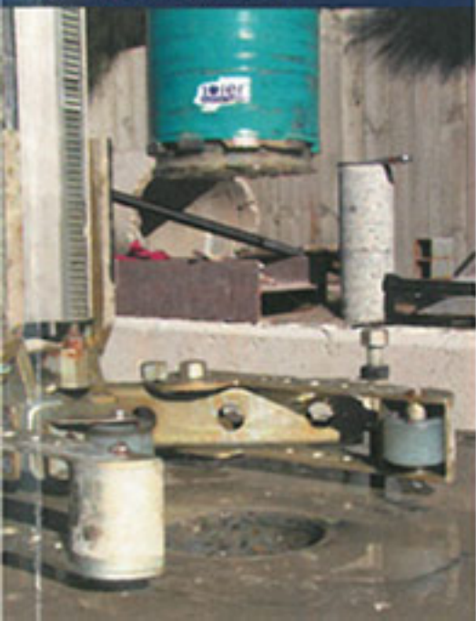
BELOW: Core Catcher System
